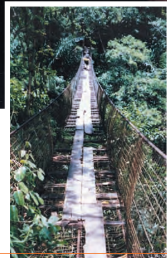
THE VILLAGE BRIDGE – IN NEED OF A LITTLE REPAIR!
