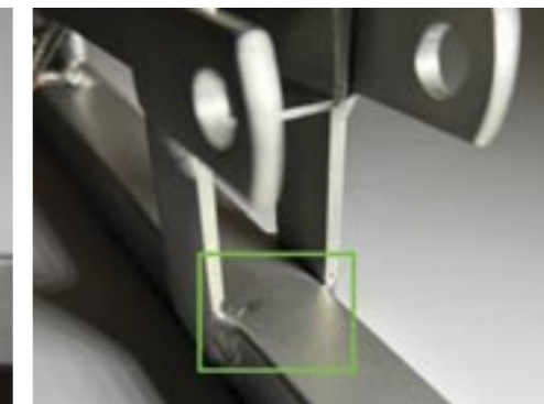
Figure 5: Inspect all welded joints and the surrounding material on both horizontal faces of the handle including corners. Pay extra attention to the area in the green box on the underside (when deployed) of the handle.
